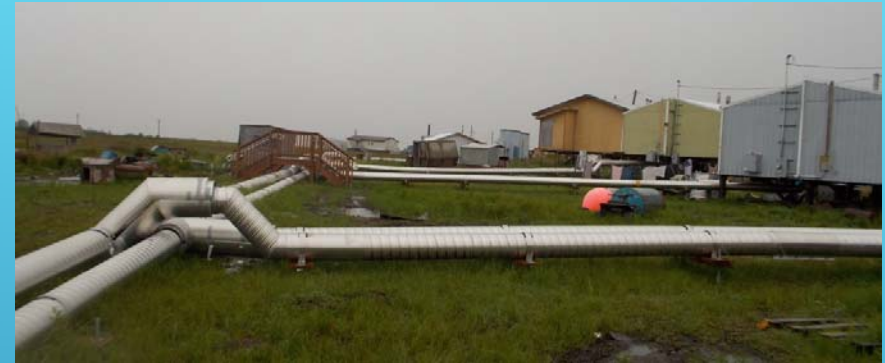
Above grade pipes in Quinhagak
