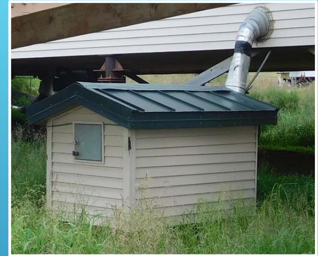
FT&H System Sewage Tank
