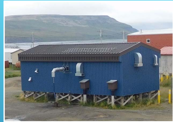
School Water Treatment Plant and Watering Point
